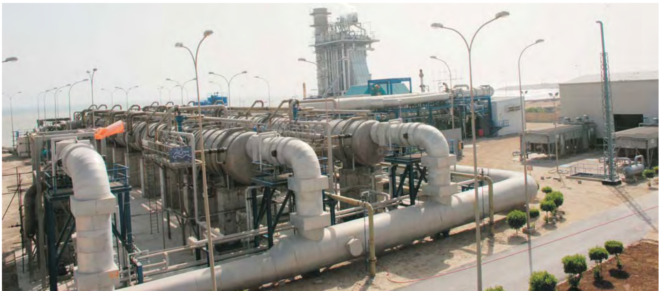
DHA Cogen Power & Desalination Plant
