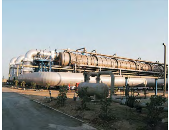
A side angle view of the DHA Power & Desalination Plant
