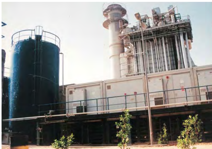
Another angular view of DHA Power & Desalination Plant
