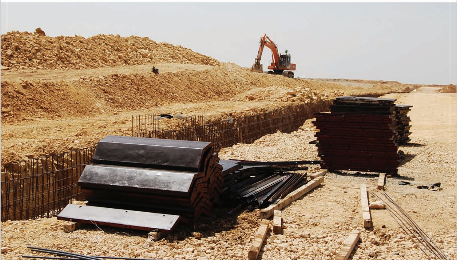
A view of DCK Directorate Building under construction at DHA City Karachi
