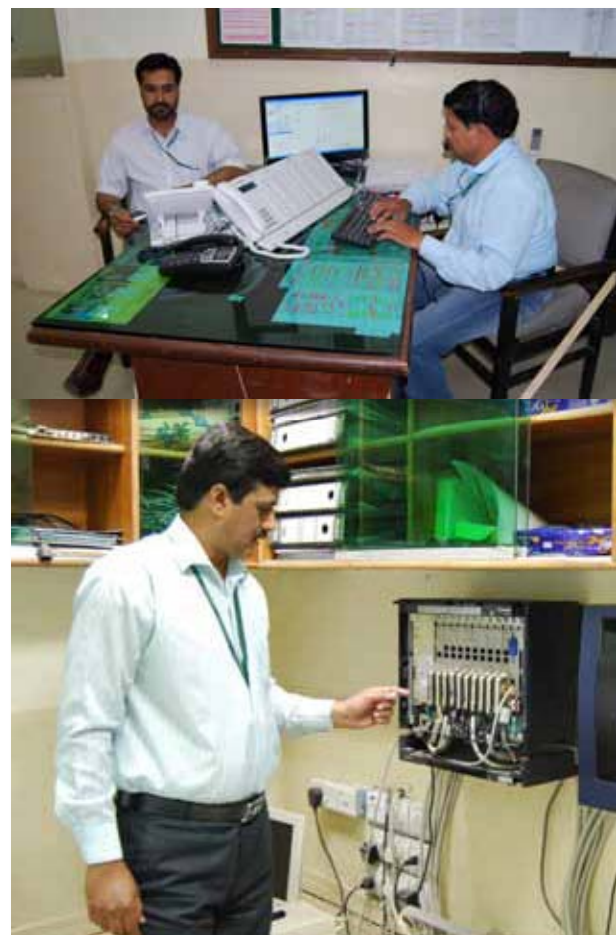
A view of New Digital Exchange installed at DHA's Main Office
