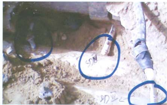
Illegal water connections
